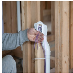
Low voltage cable, approximately 150mm tails
